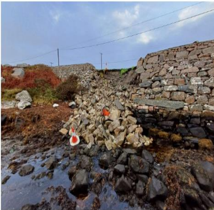
ROAD EMBANKMENT FAILURE, CNOC, LEITIR MEALLAIN
