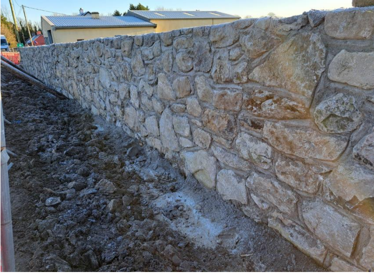
CONSTRUCTION OF A STONE WALL IN LABANE TO FACILITATE A NEW FOOTPATH.
