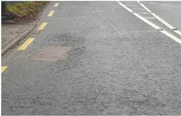
BEFORE ROAD REPAIRS N83 DUNMORE
